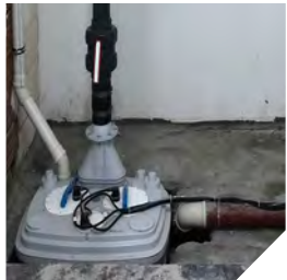
-1. kat zeminine kurulan SANICUBIC 2 VX
